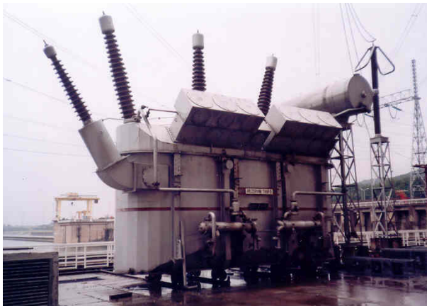
Fig. 1. A transformer of the power plant Djerdap 1
